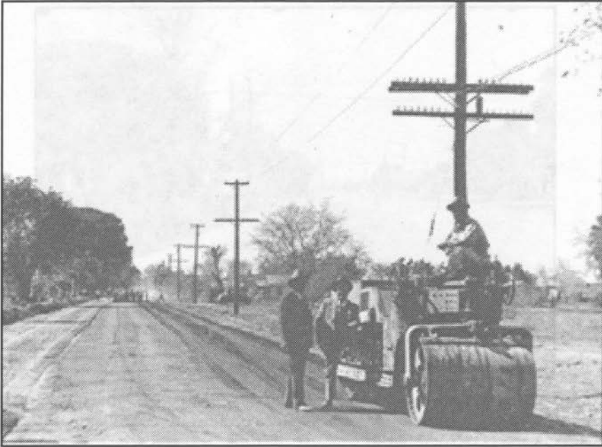
Figure 12. CWA road paving project on Thomas Road, Phoenix. Arizona Department of Library, Archives and Public Records, History and Archives Division, Phoenix, #98-3335.
