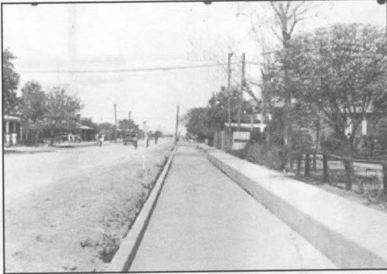
Figure 14. Drainage system project, Douglas. Arizona Department of Library, Archives and Public Records, History and Archives Division, Phoenix, #98-3583.
