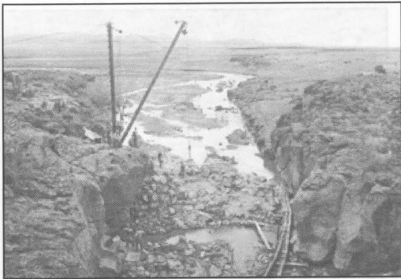
Figure 19. Sullivan Dam under construction, Yavapai County. Arizona Department of Library, Archives and Public Records, History and Archives Division, Phoenix, #98-4085.
