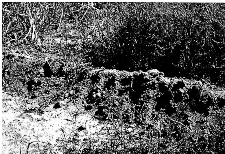
Figure 4.3. An example of a small earthen diversion dam or berm in the vicinity of the Río Sonora (photograph courtesy of Paul and Suzanne Fish).
