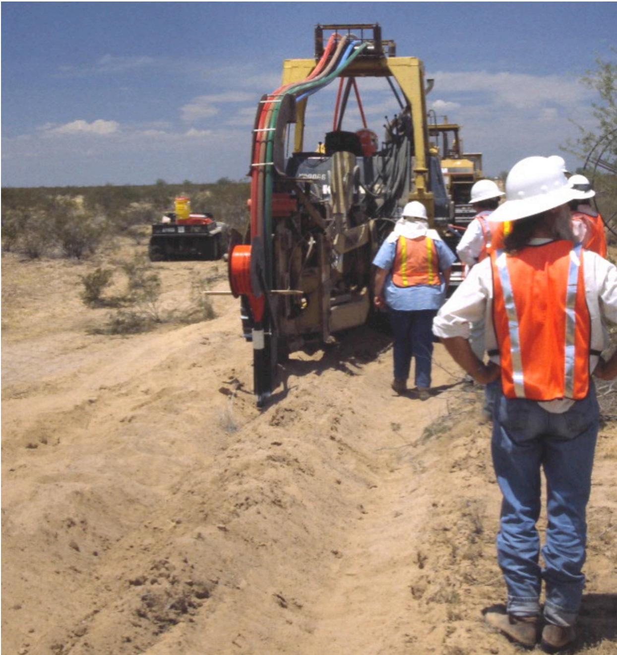
Figure 1. The area of potential effect for direct impacts associated with this fiber-optic installation includes the ripped area containing the conduit (lower left), areas crossed by construction equipment (center), and room for support vehicles, such as the all-terrain vehicle, to maneuver (left).
